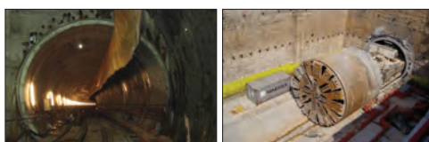
Example of tunnel under construction using a tunnel boring machine (right). Exemple d'un tunnel en construction utilisant un tunnelier (photo de droite).
